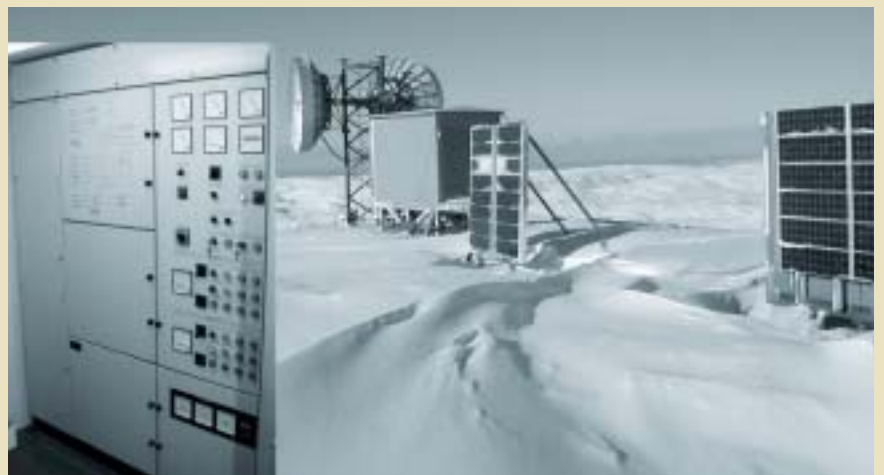
SystemTeknik A/S has been chosen to supply radio station control equipment for the whole of Greenland. The picture shows such station, with its panels, generator and transmitter equipment.
